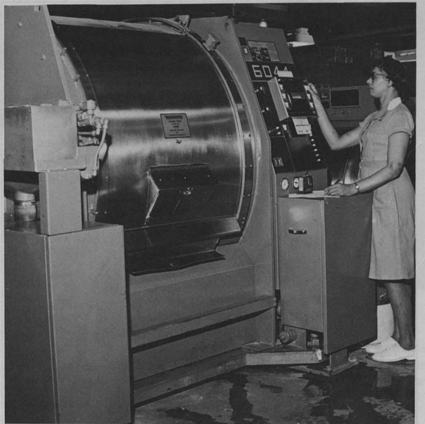
The Hospital laundry has entered the computer world with the recent addition of three new 400-pound washerextractors and modernized folding equipment. With the installation of the new machines over 8,000 pounds of laundry can be handled in a much easier and faster method. Checking out the computer on one of the new washers is Mrs. Georgia Mae Naylor, Utility Worker Grade 4.
