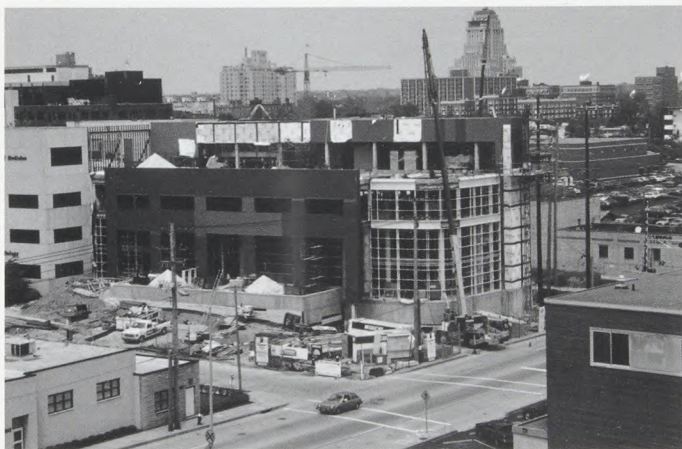
The Mallinckrodt Institute of Radiology Imaging Center at the corner of Scott and Taylor avenues is nearing completion. The three-story facility with its distinctive east facade of green-tinted wraparound glass officially opens November 11, 1994.
