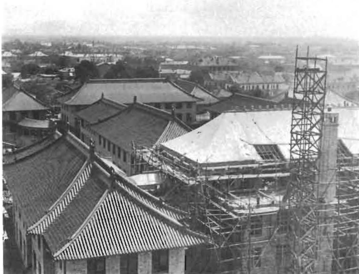
Construction of the Peking Union Medical College, ca. 1918. From the Cowdry Collection, WUMS Archives.
