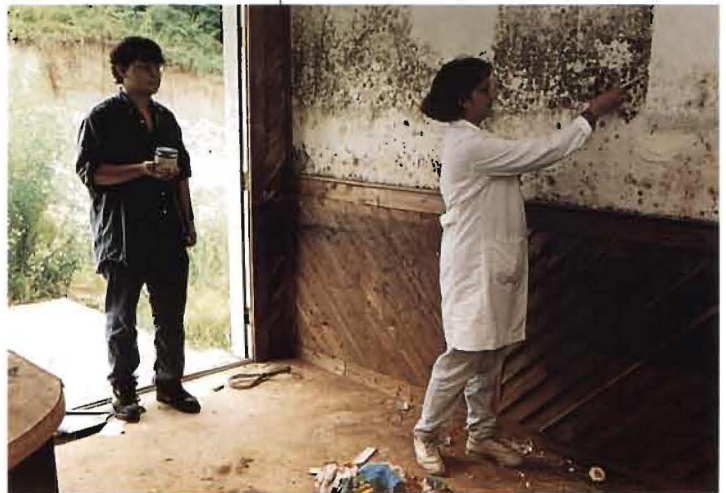
Anu Dixit, Ph.D., right, collects mold samples from an interior wall of a flood-ravaged, abandoned house in Imperial MO. Dixit and research assistant Harley Wieselthier, left, are studying the health effects of continual mold exposure.
