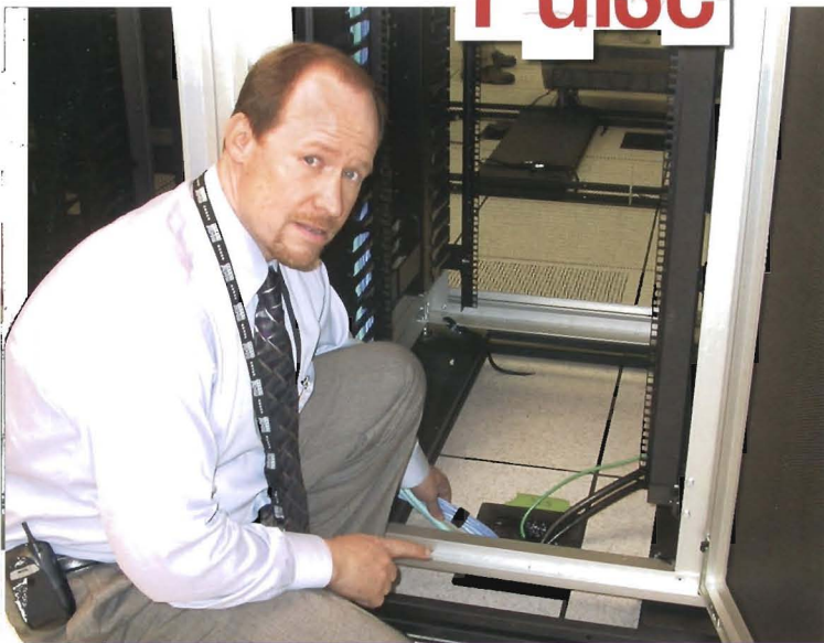
Tim Brooks, director of information systems and HIPAA security at the Bernard Becker Medical Library, points out the seismic mounts and flexible cable access, two of the features that protect critical resources at the new Medical School Business Continuity Center, located on the North Campus.
